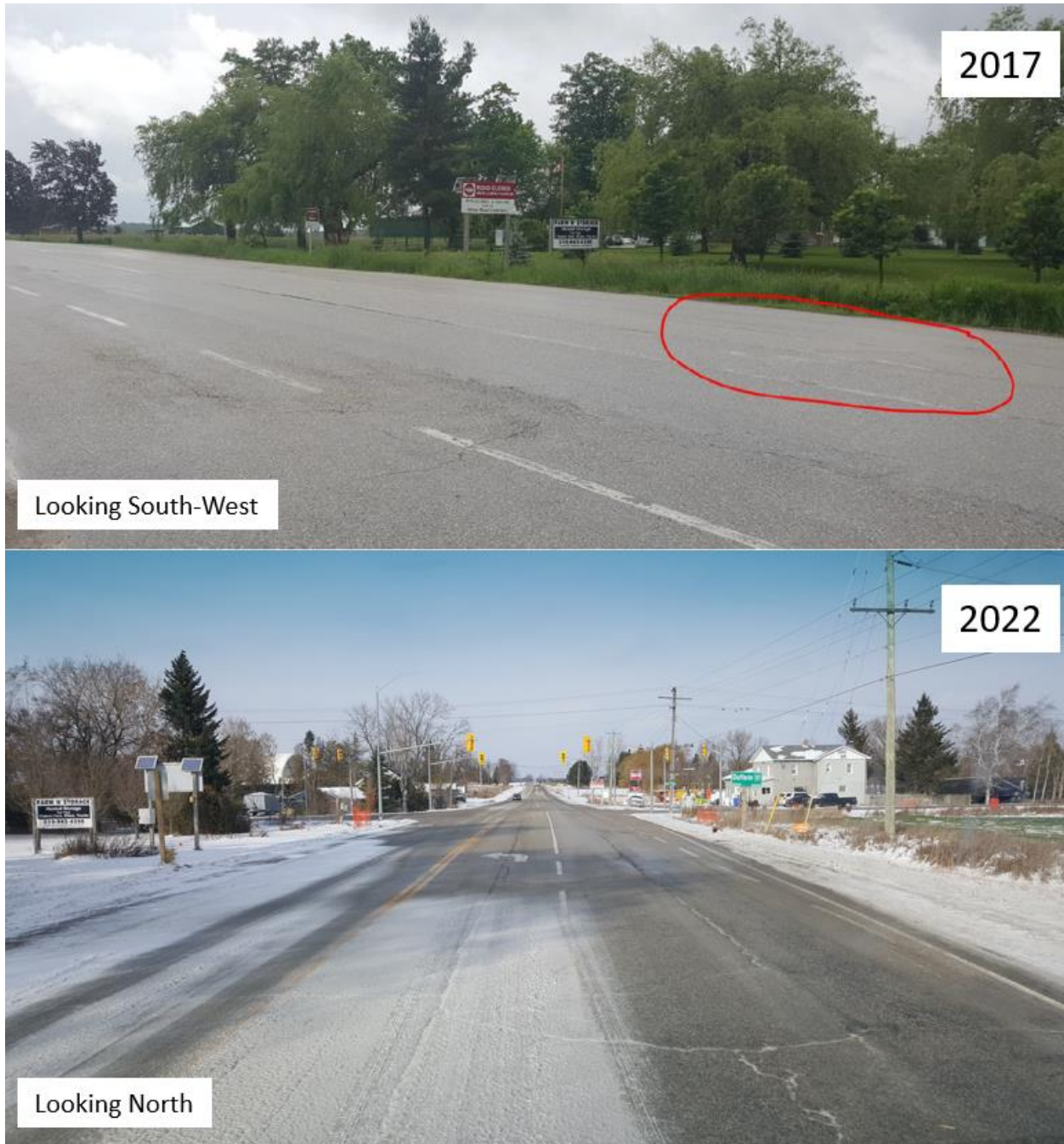
Exhibit 23: Dufferin Road 17 @ Dufferin Road 124 Northbound Trailing Left-turn Arrow
