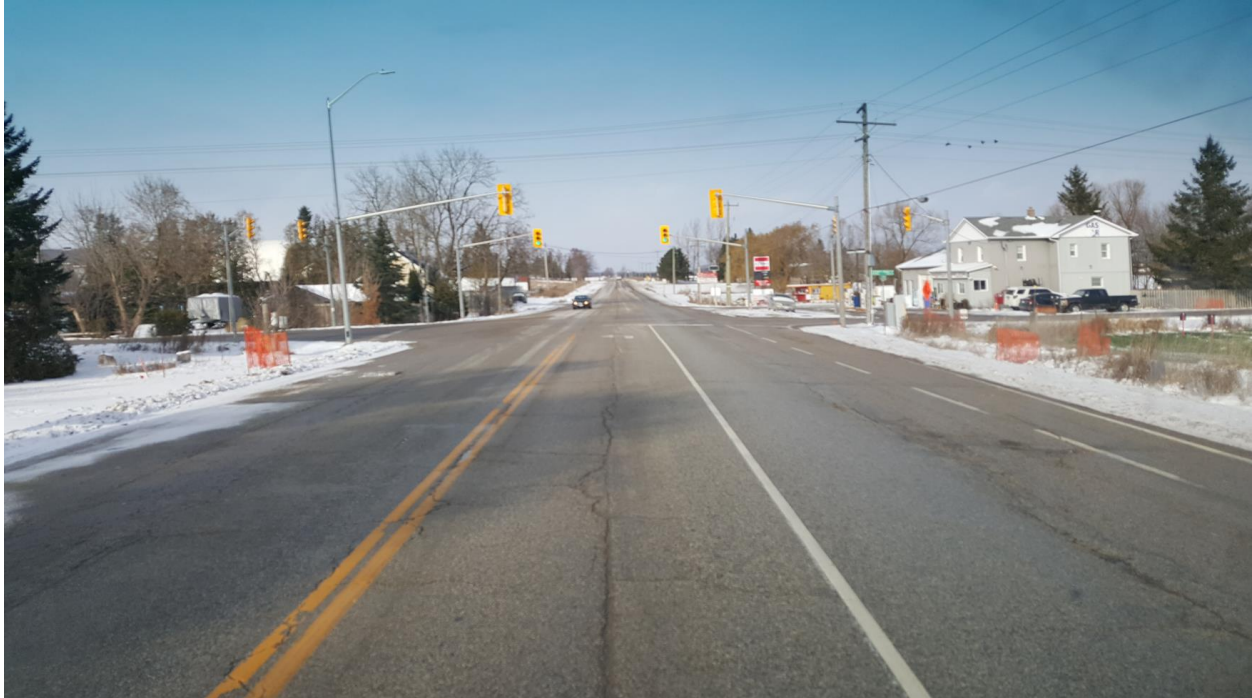
Exhibit 28: Longitudinal Cracks along Dufferin Road 124 Looking North, 2022
