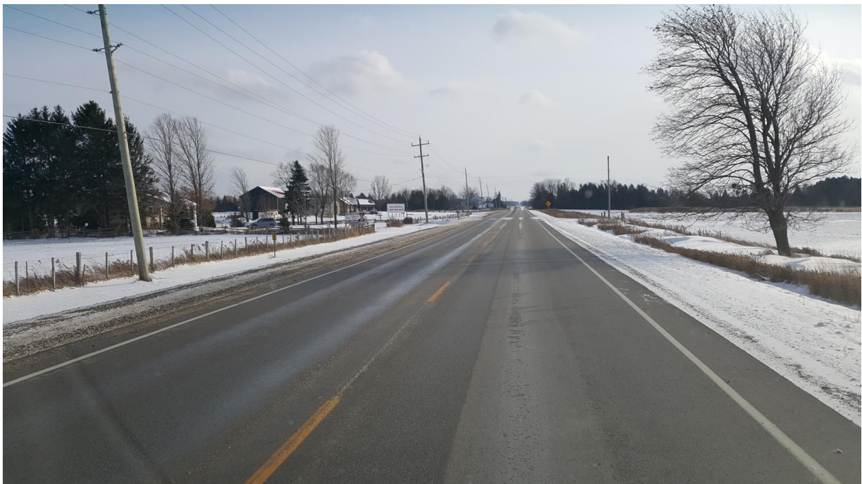
Exhibit 27: General Pavement Conditions along Dufferin Road 124 Looking South, 2022
