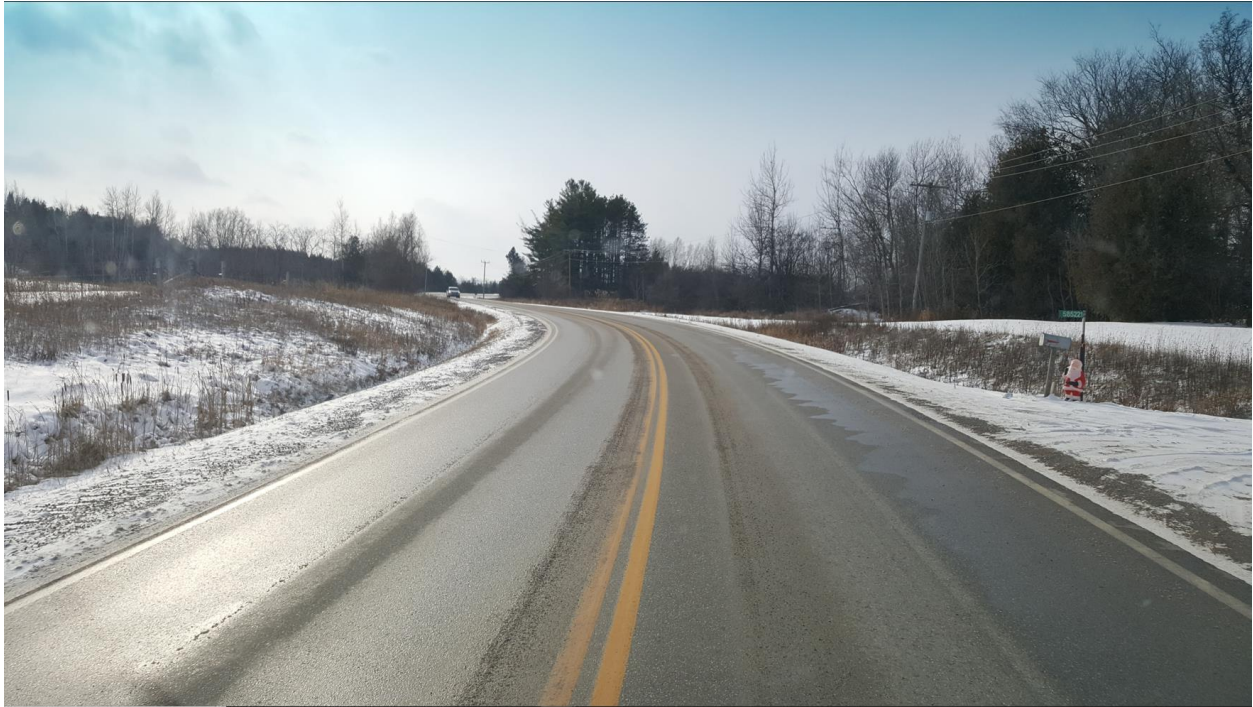
Exhibit 26: Pavement Conditions along Dufferin Road 17 Looking West, 2022
