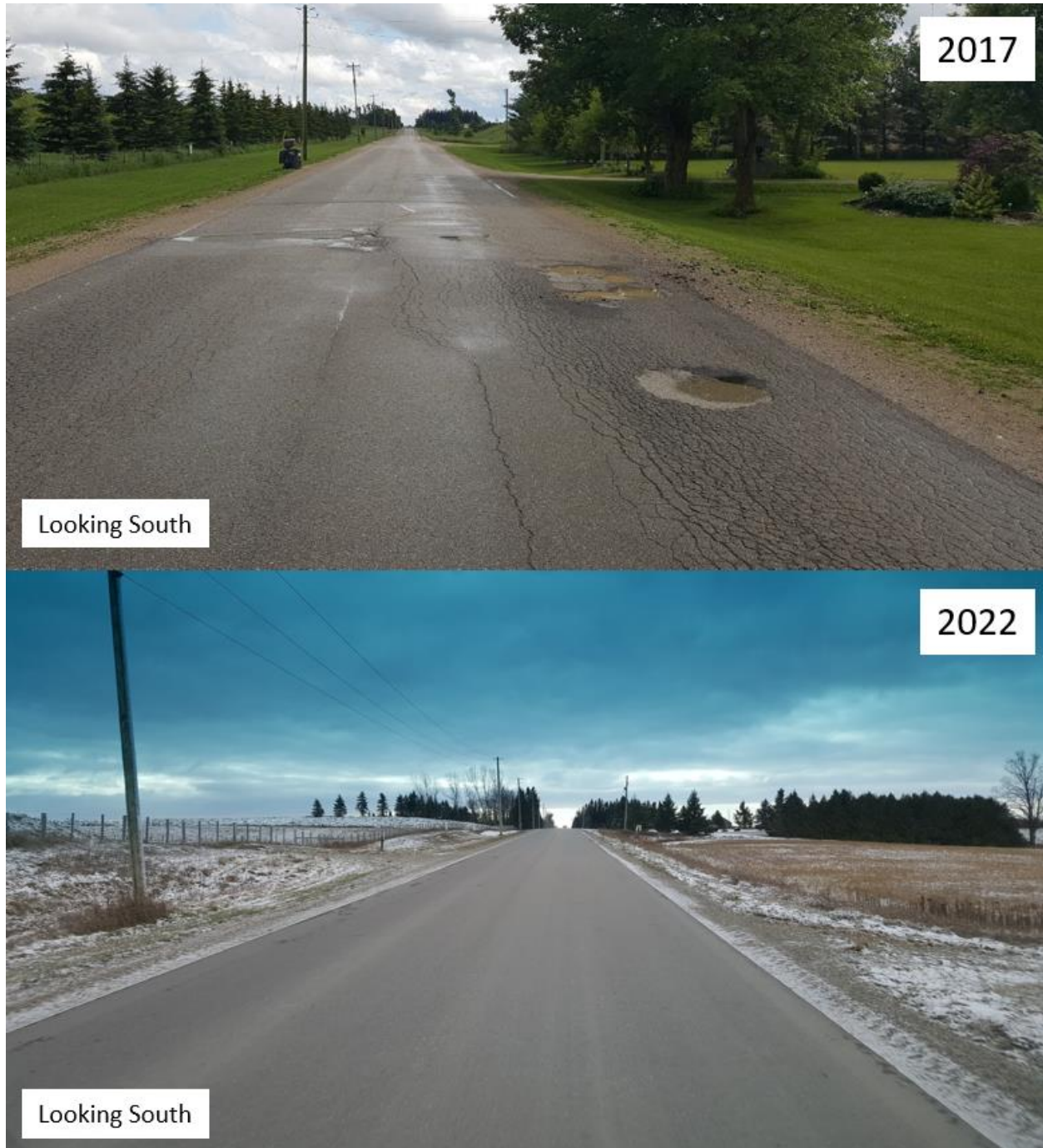
Exhibit 25: Potholes on 4 th Lines and Pavement Conditions along 4 th Line
